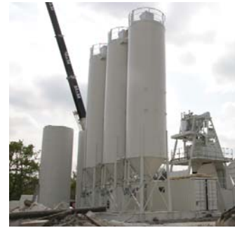
Mobile plant at Sellafield.
